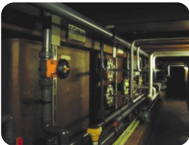
▲ Picture 1: Dry cellar – no aggressive fumes attack the sensitive equipment
