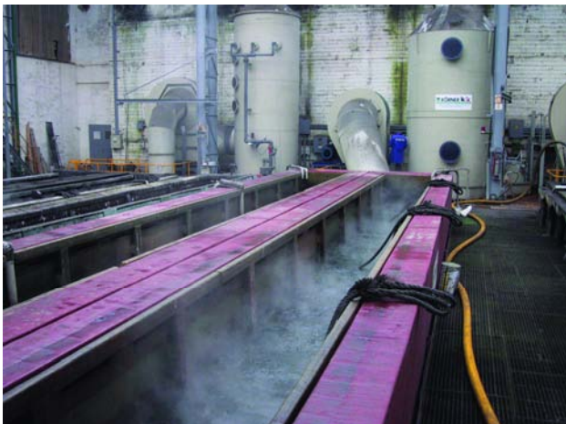
Picture 1: Pre-treatment tank with lateral fume extraction channels: fumes are caught, when tubes are immersed
