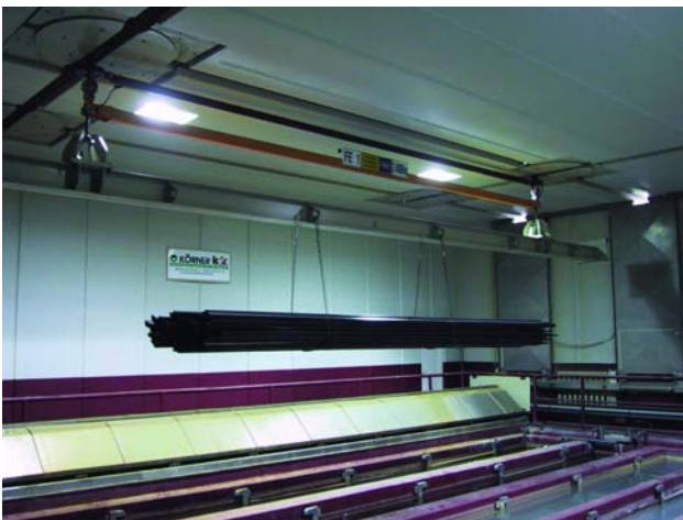
Picture 5: Encapsulated pickling area: only chains or ropes are exposed to aggressive air and crane units are running outside
