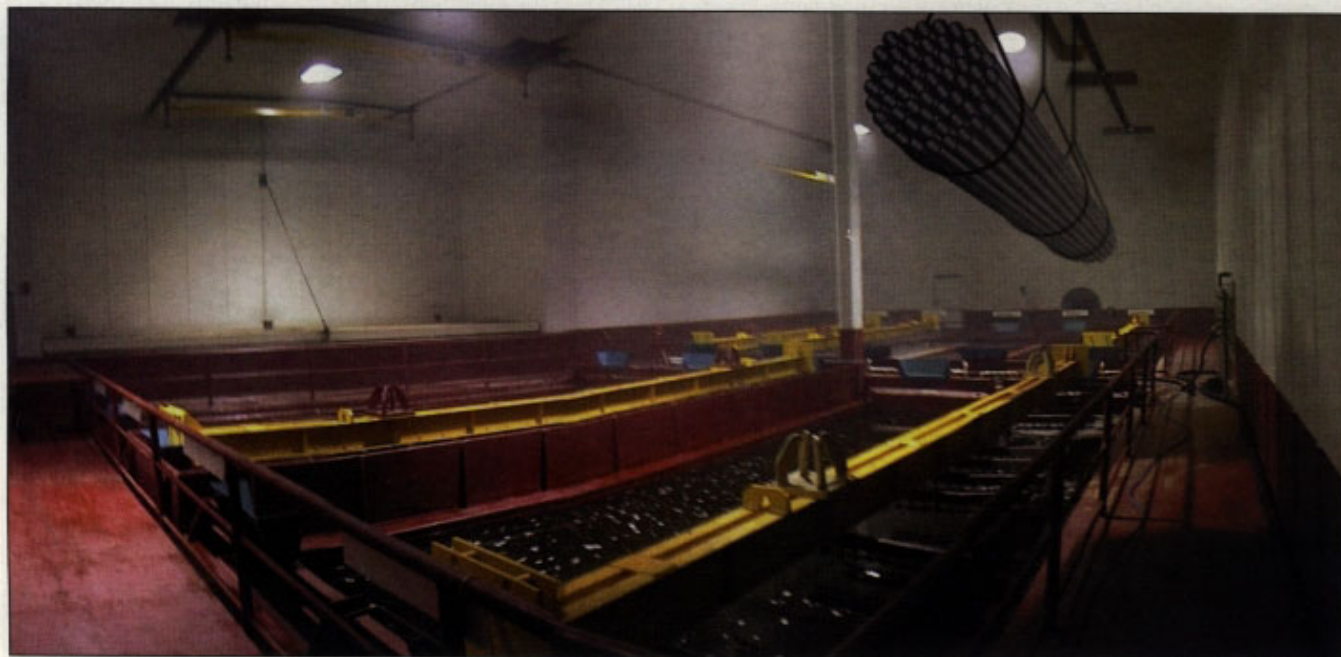
Figure 3. Inside the encapsulated pickling area, where the transport system operates fully automatically. Note no operating personnel inside the enclosure
